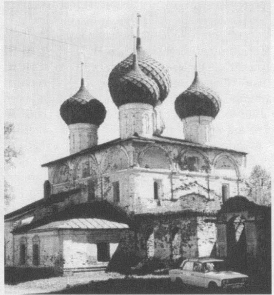
Fig. 14.219. A typical Russian church of the XVII century. We see the northwest view of the Nikolskaya Church, Nikolo-Ouleymenskiy Monastery, Ouglich. Most Russian churches of the XII-XVI century are supposed to have been constructed in the same manner as this one.
