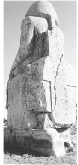
Fig. 19.119. The right Colossus of Memnon (rear view). There is a large Orthodox cross on the back of the throne. Incidentally, new cracks have appeared on the statues over the last couple of years – we don’t see them on the photographs taken a few years before. Photograph taken in 2000.
